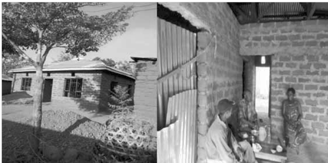
Plate 3: A Moderate House under Construction Built by a Woman Involved in Vegetable Business and a Family in a House
