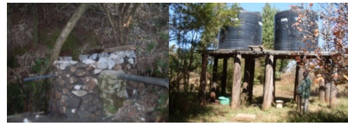
The water source Water reservoir
